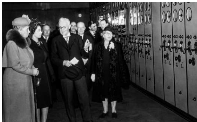
(Caption: The Queen, then Princess Elizabeth, visiting Battersea Power Station in April 1946 with her Grandmother Queen Mary (left), for a special tour inside the Power Station and Control Room A – credit Simon Webster/Alamy Images)
