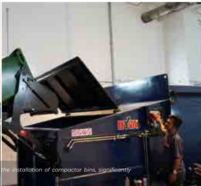
KL East Mall strengthened its waste management practices through the installation of compactor bins, significantly reducing waste volume and improving operational efficiency
